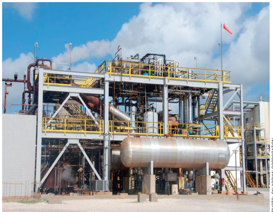
SO 2 Clean sulphur dioxide plant at Port Neches, Texas.
